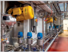
The mixers are in a new facility
