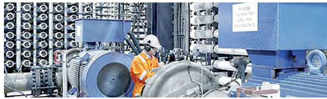
ABB says its Energy Snapshot gives a new perspective on maintenance costs
