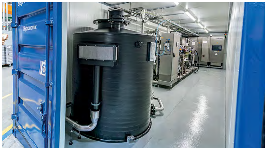
In the shipping container, all the machine components were ready and in place in time for the FAT at the end of March
